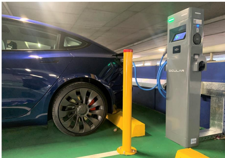
Public place EV charging. Parramatta Station Car Park, Wentworth Street
